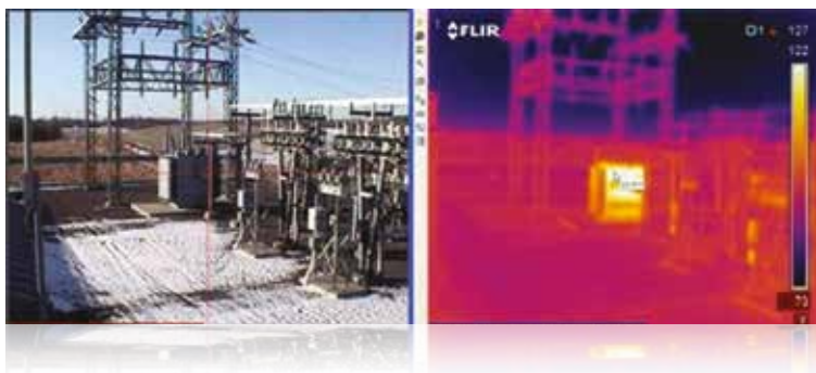
Figure 10. Visible light and IR images of a substation showing a transformer with excessive temperature.
